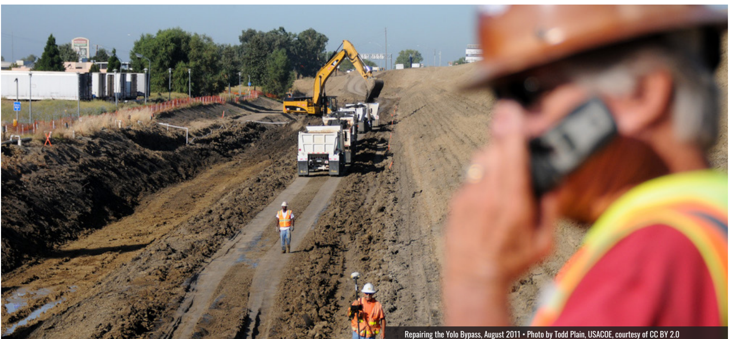
Repairing the Yolo Bypass, August 2011 • Photo by Todd Plain, USACOE, courtesy of CC BY 2.0
